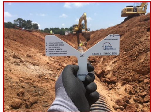
An example of sloping and a Trench Slope Tool for Type C soil
