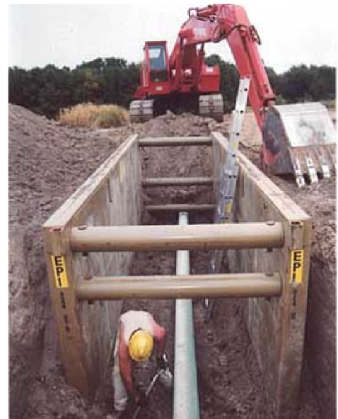
An example of a trench box used during water line installation; safe, neat, and efficient
